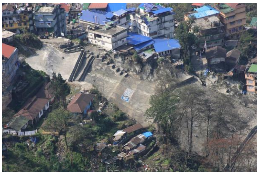
Photo Plate 7: Treatment of Mangan landslide completed under LRMS project of NDMA & SSDMA.
