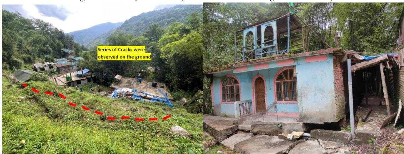
Photo Plate 1: Lumsey Subsidence Zone, Gangtok, Sikkim
