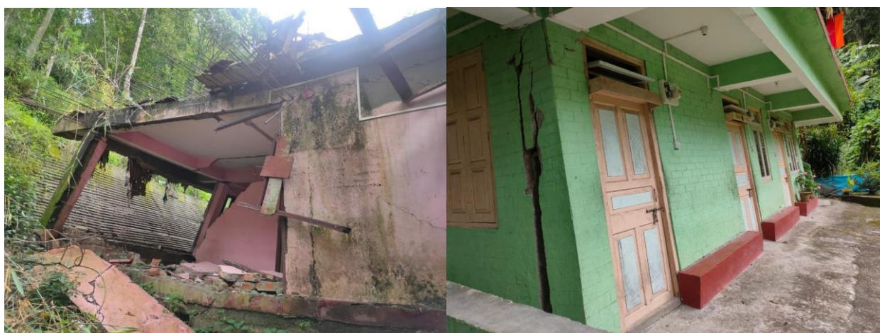
Photo Plate 2: Lumsey Subsidence Zone, Gangtok, Sikkim
